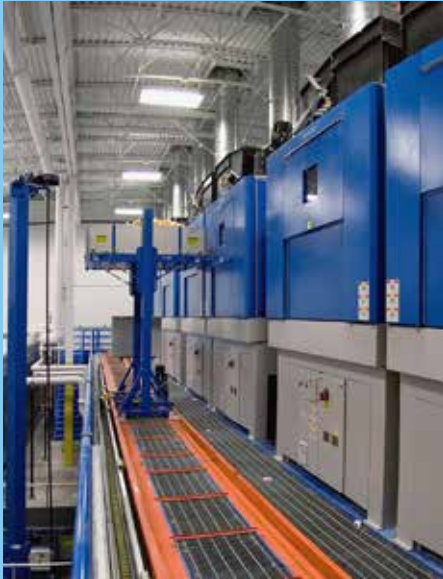
DT 140 Plus Dryers have the same footprint as its predecessor and can be arranged in a bank to be fed by shuttle conveyors.
