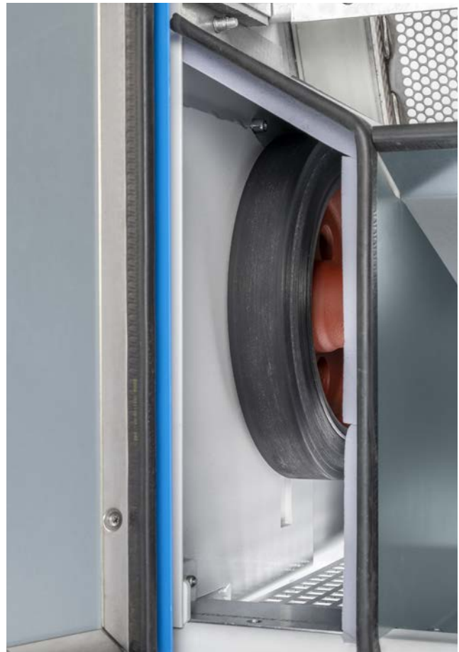
The drive wheels are now being protected directly from the hot air stream.
