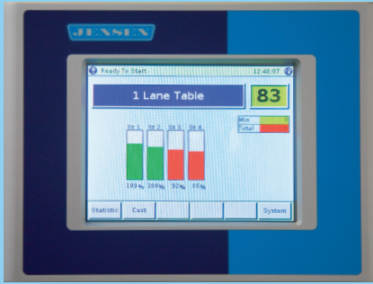
17 Jentrol MMI PLC and control system with touch screen
